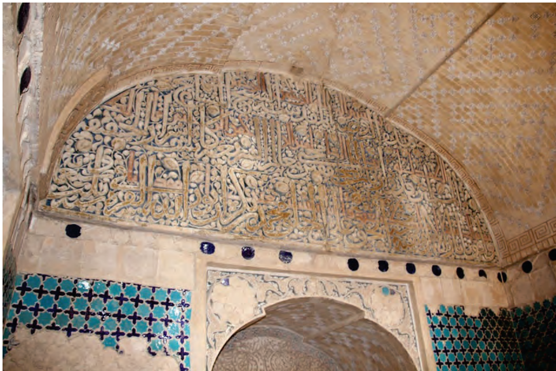
Img. 5: Pir-i Bakran mausoleum burial chamber; ceiling – the khatt-i banna'i (first stage); stucco inscription dated 1303-04 (second stage), which conceals earlier revetments in stucco and cut ceramic inscription (first stage); moulds of tile frieze from the first decorative stage; star and cross tiles (third stage). (Grbanovic 2018)
